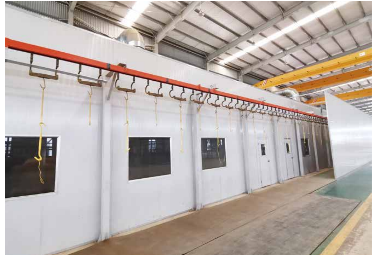
结构件喷漆线 Structure Painting Line
